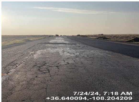
BEFORE: Cracked surface on paved road.
