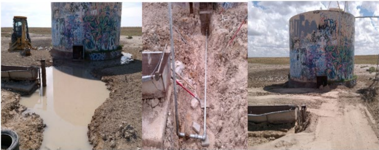
Standing water had to be drained, pipes and stop n waste value replaced at Windmill No. 513-1 in Whitecone Chapter .
